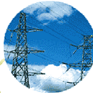
Aerial Power Cables
