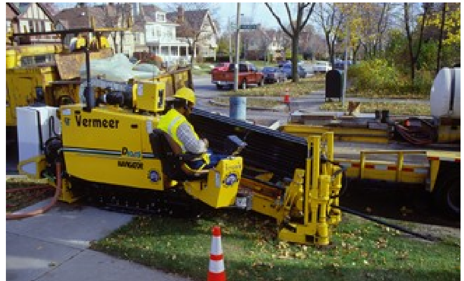
Figure: Non-intrusive deployment of cables under pavements using horizontal directional drilling (Source: Vermeer).
